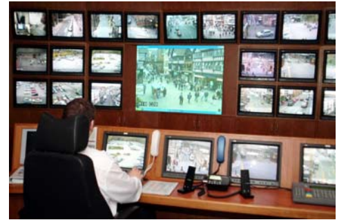
The video wall in Chester City Council's Control Room
